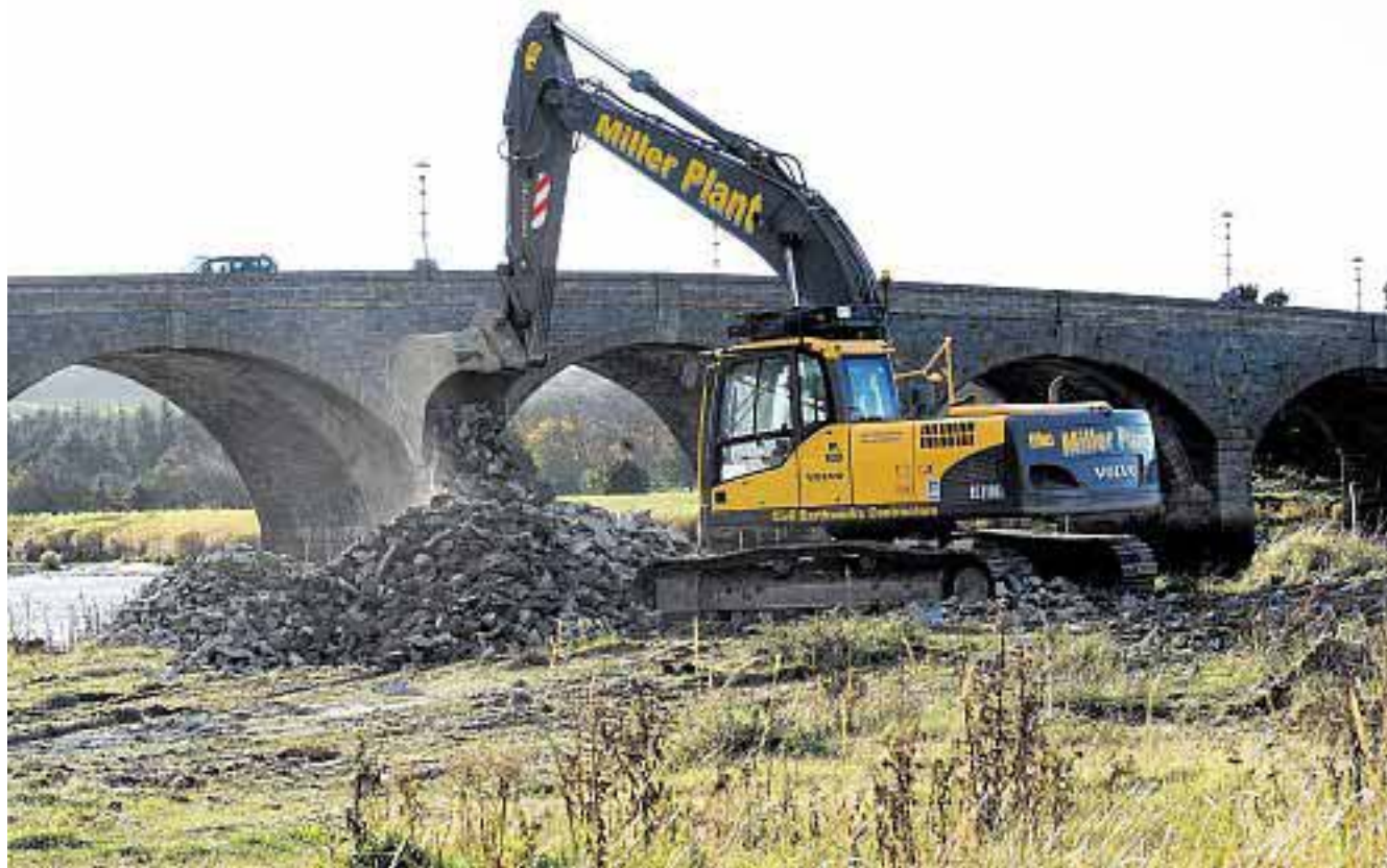
HISTORIC SPAN: Repairs to Banff Bridge will see heavy rocks placed round the structure's supporting piers
