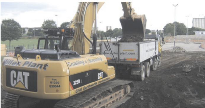
Digging in: The company starts on its earthworks contract for the Queen Mother Library.
